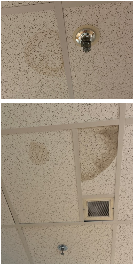
Figure B.5. Examples of stained ceiling tiles at the healthcare center. Source: Photos taken by OIG inspector.
