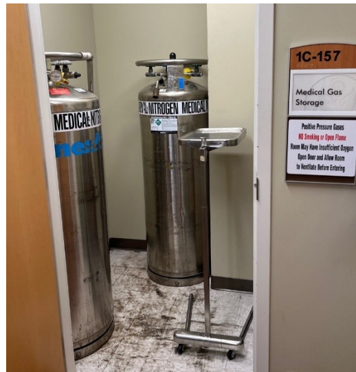
Figure B.6. Unsecured nitrogen tanks in the dermatology clinic at the hospital. Source: Photo taken by OIG inspector.
