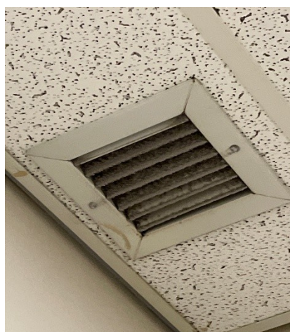
Figure B.2. Examples of dust on ventilation grills observed in both the hospital and healthcare center. Source: Photos taken by OIG inspector.
