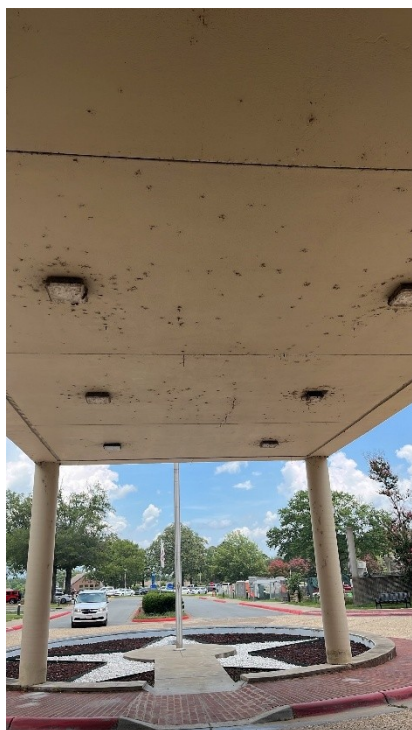
Figure B.1. Stained ceiling with hanging mineral deposits above the passenger loading zone at the main entrance of the healthcare center. Source: Photo taken by OIG inspector.
