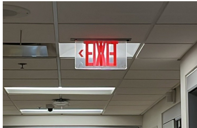
Figure B.2. Difficult to read exit sign.
